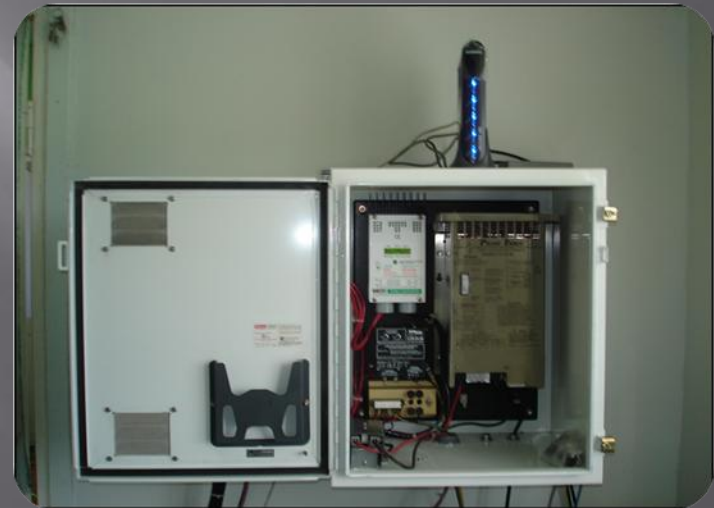
Main power control and management unit
